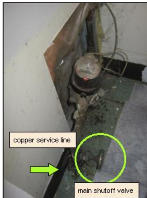
water meter and main
