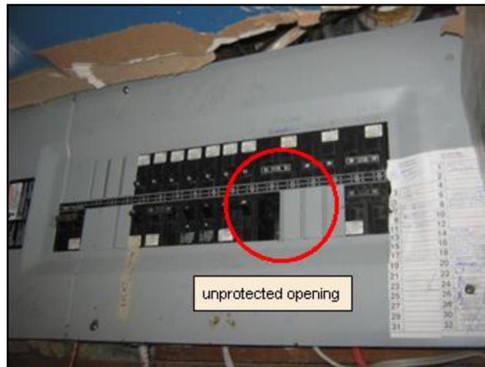
main service panel
