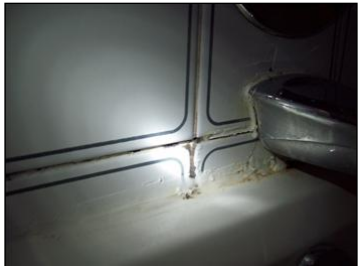
Deteriorating tile. Some mildew noted.
