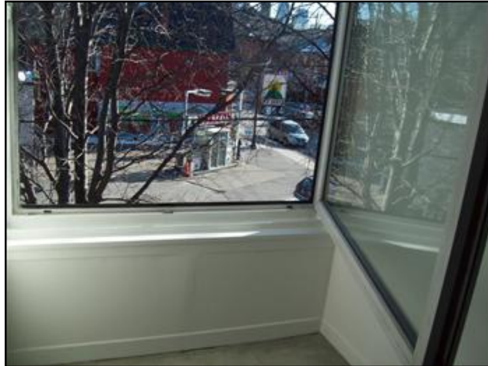
Caution. Second storey window. Fall hazard.
