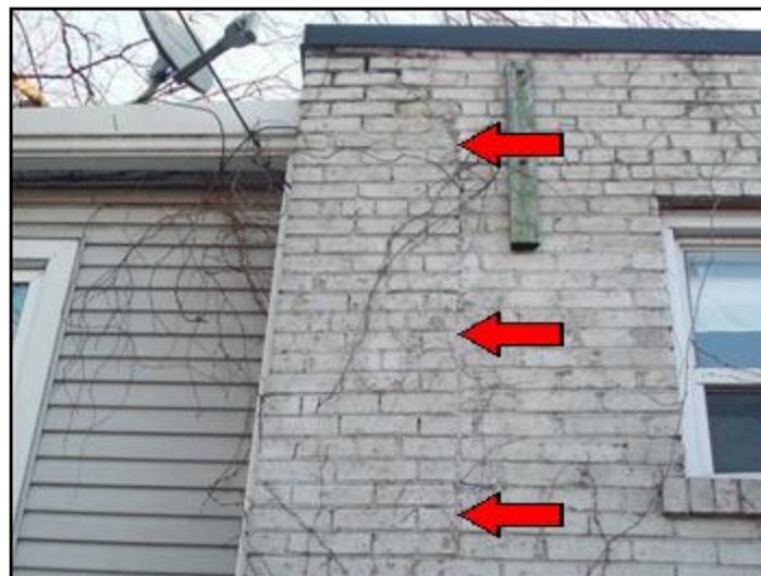
Mortar Deterioration in joints
